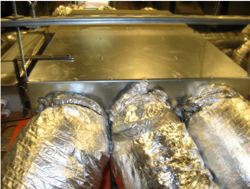
Ducts entering unit at rear.
